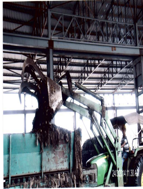
COMPOST PROCESSING UNIT
