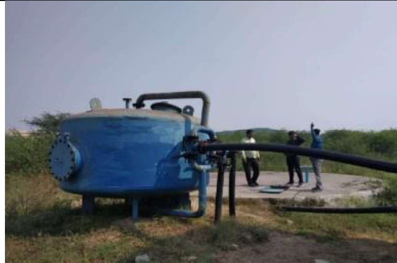
Pressure filter of capacity 45 cum/hr installed to supply treated mine water to pond at Sakhari village
