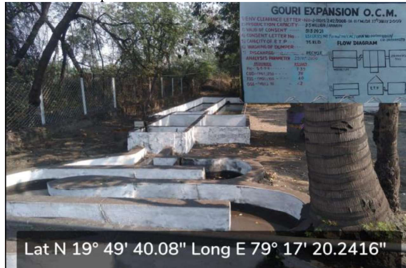
Effluent Treatment Plant
