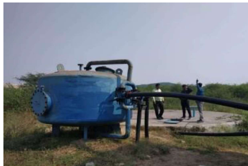
Pressure filter of capacity 45 cum/hr installed to send treated mine water to pond at Sakhari village
