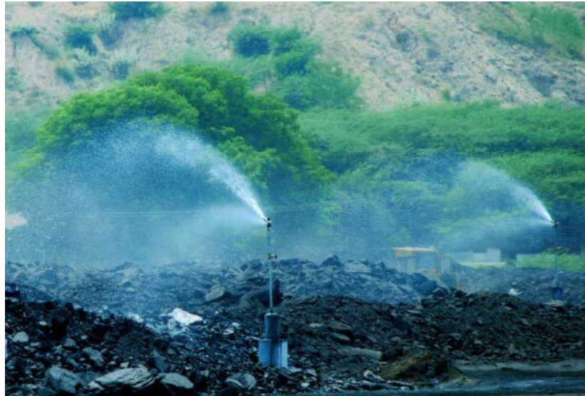
Rain guns at coal stock yard
