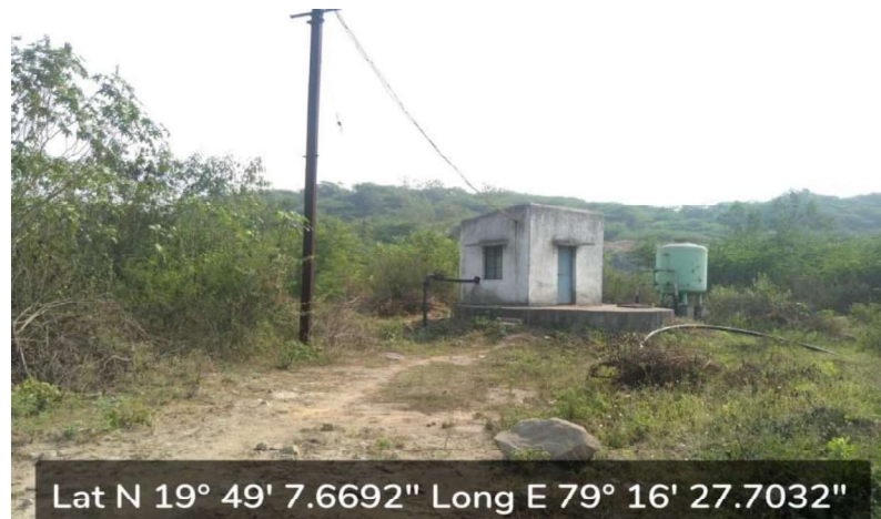
Pressure filter of capacity 22.5 cum/hr installed to supply treated mine water to Charli, Nirli villages.
