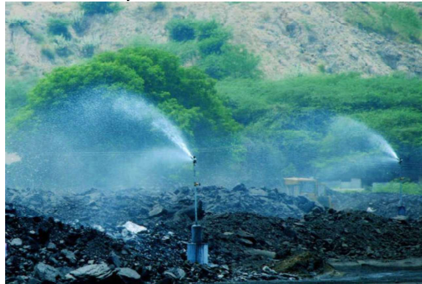
Rain guns at coal stock yard
