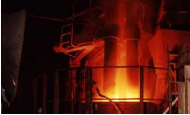
Electric Arc Furnace
