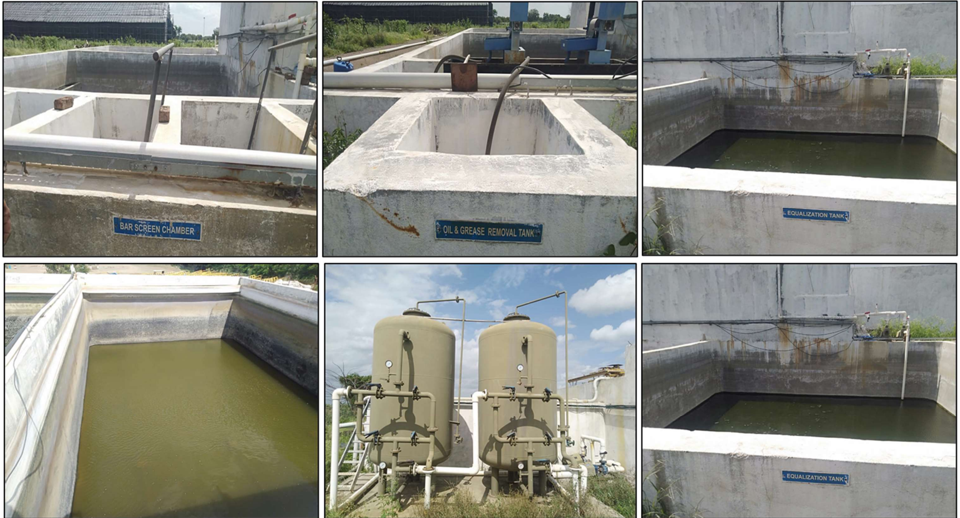
Figure 3 Existing Sugar Factory ETP Units
