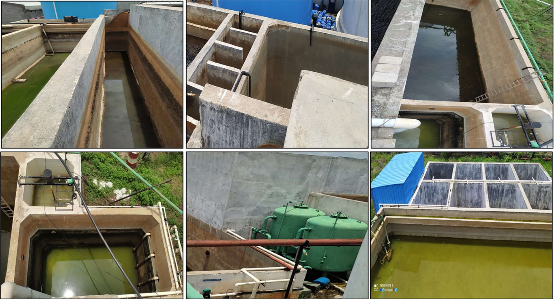
Figure 6 Existing Sugar Factory CP Units
