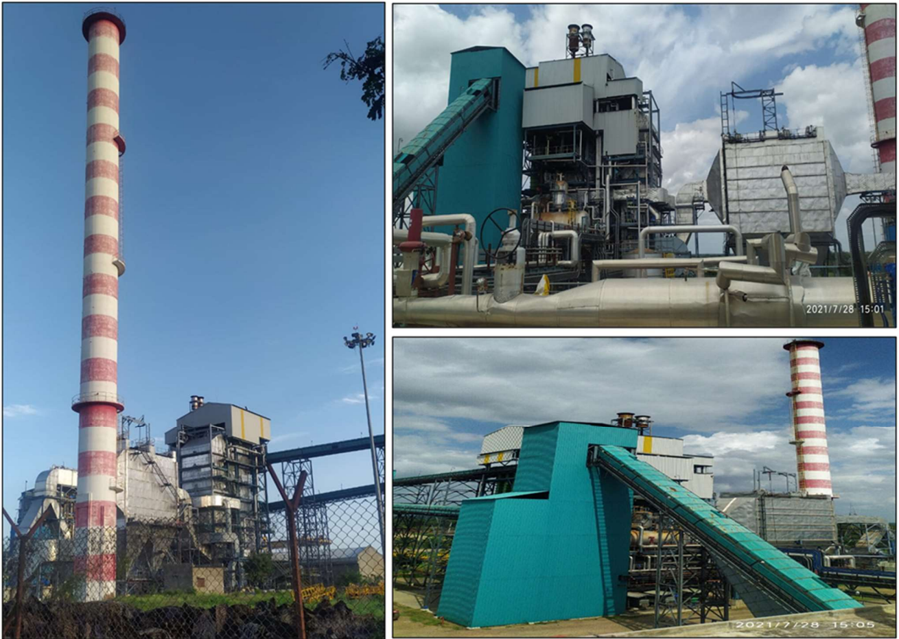
Figure 10 Existing Boiler & APC Equipments
