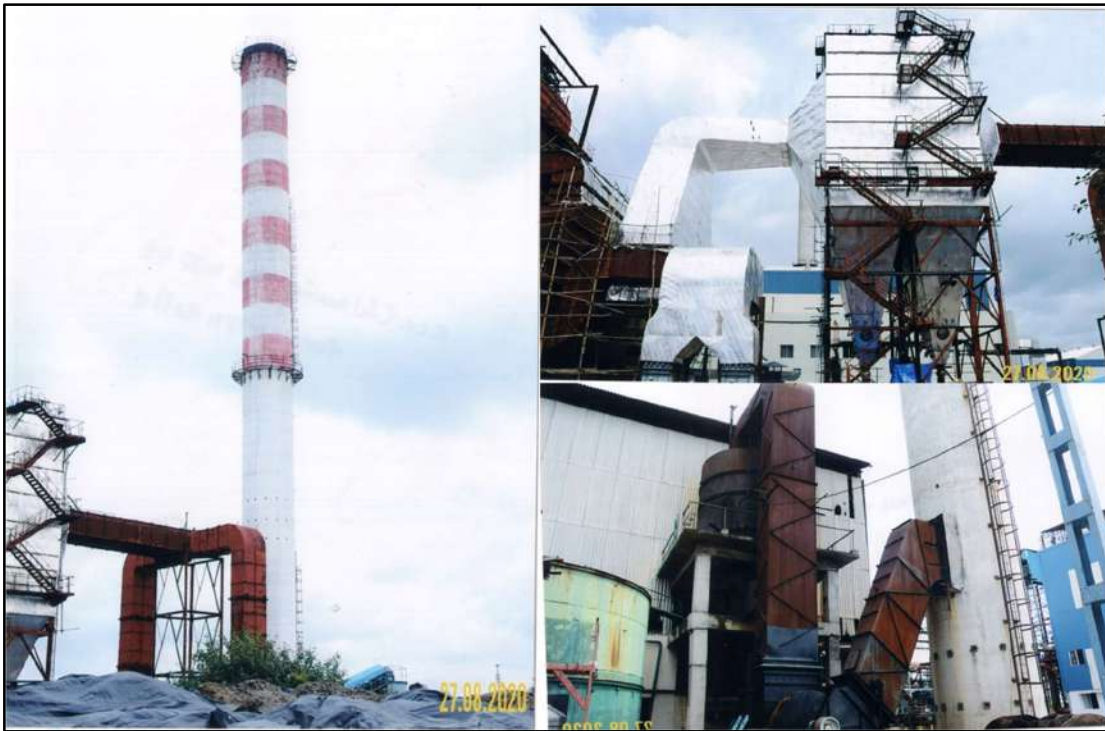
Figure 8 Existing Boiler & APC
