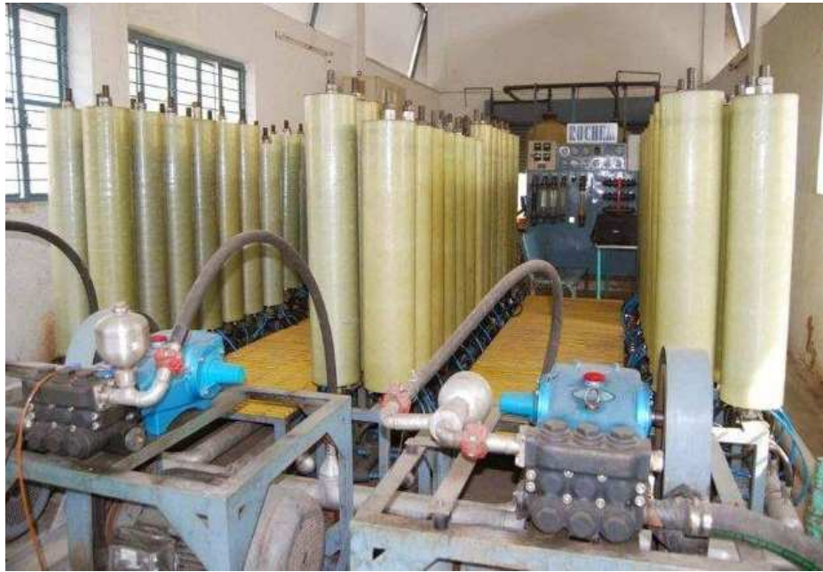
REVERSE OSMOSIS PLANT
