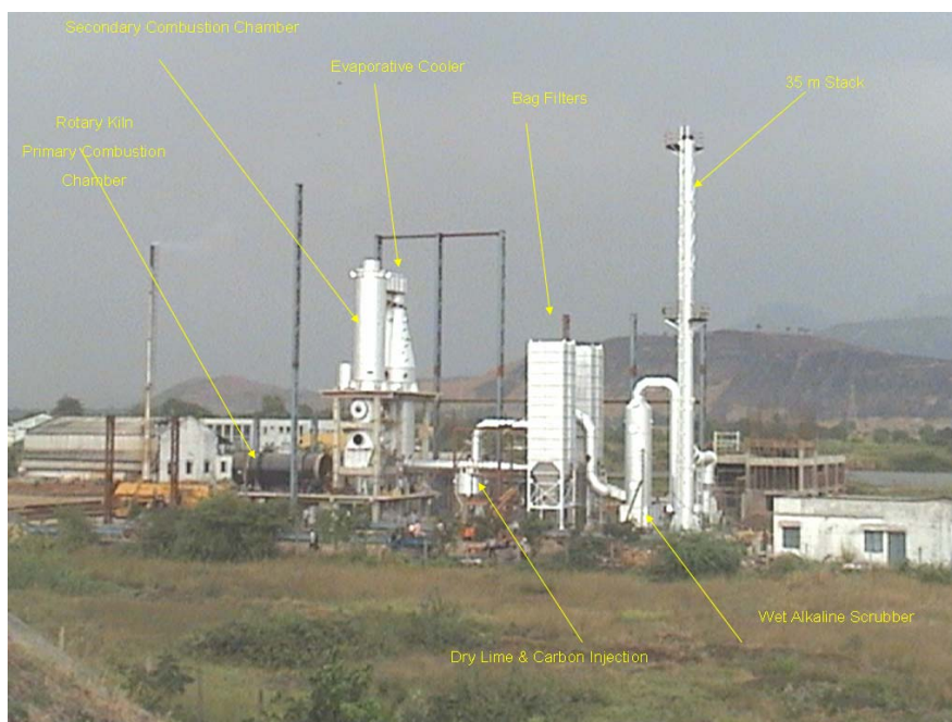
Units of the incinerator provided at MWML Taloja
