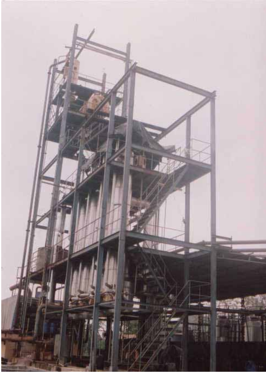
M/s. Danube Fashion Ltd., Murbad Zero discharge Multiple Evaporator system.
