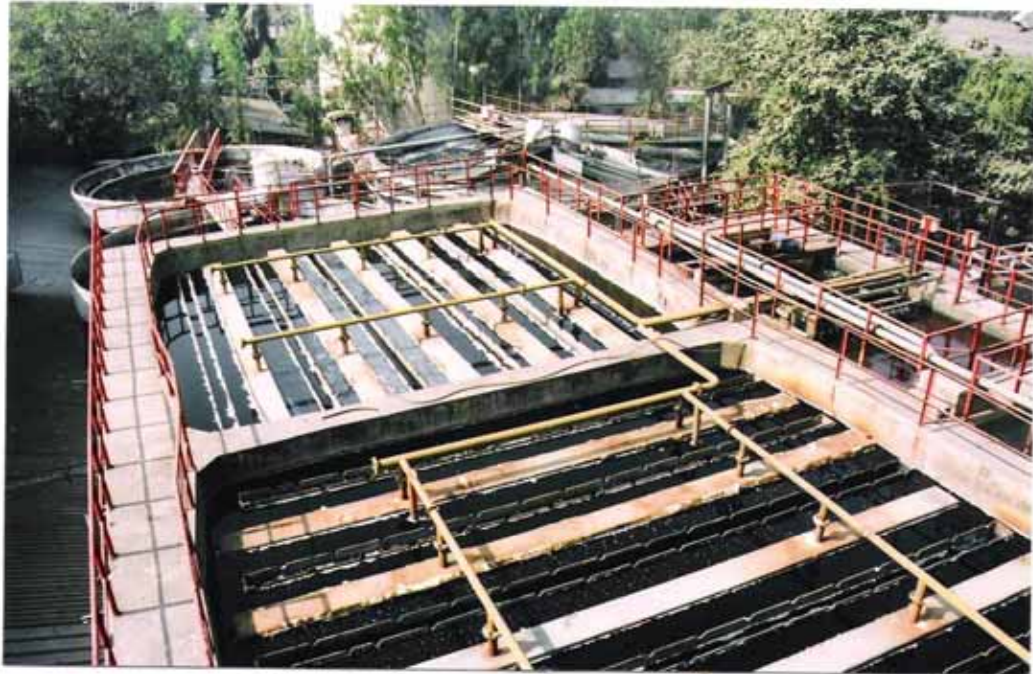
Photograph Showing ETP Unit
