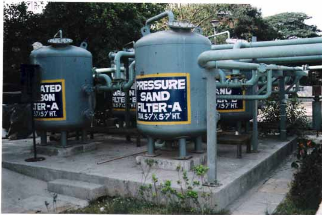
Photograph Showing ETP Unit
